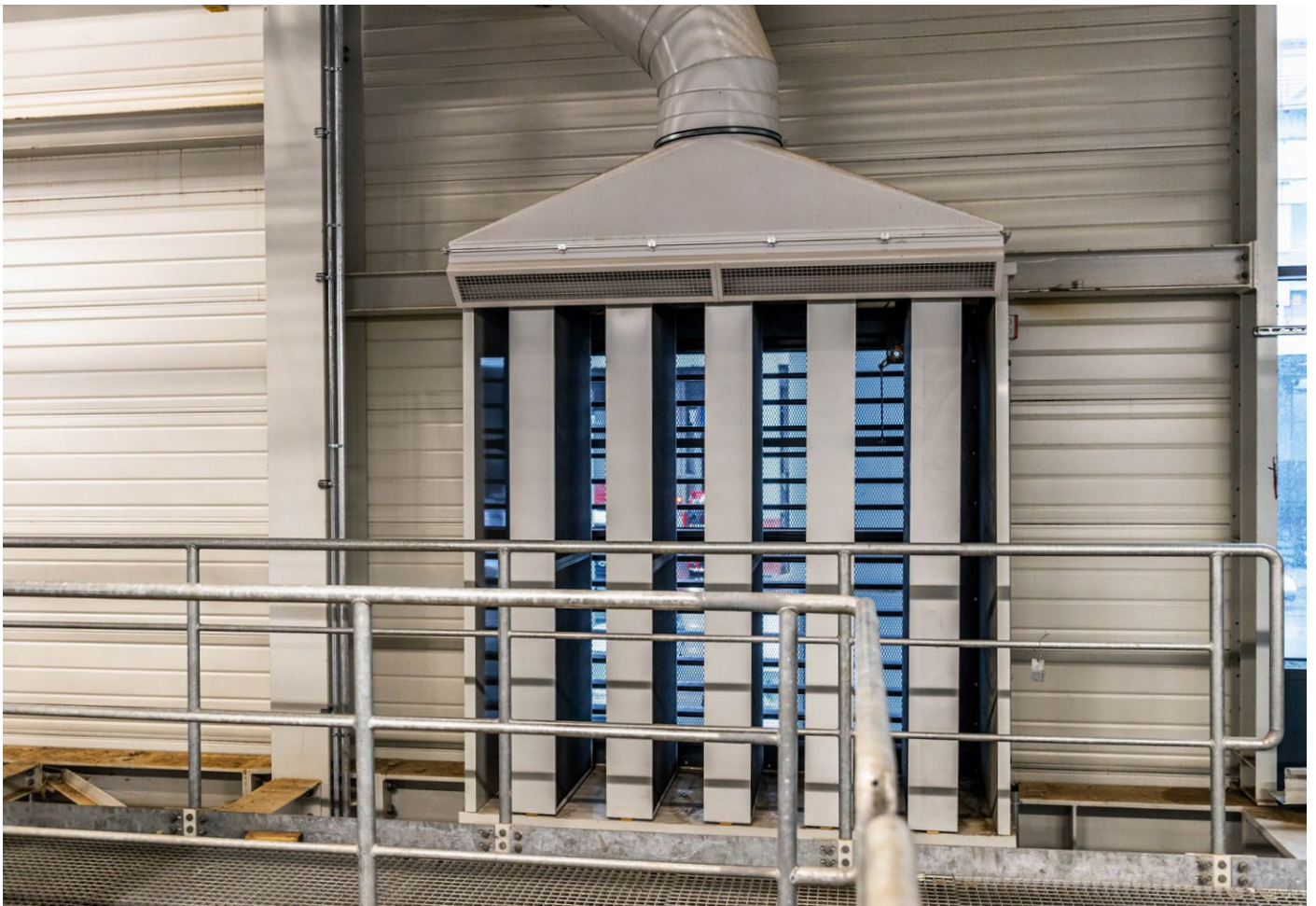
Warm air mixing system to increase the supply air temperature in winter.
